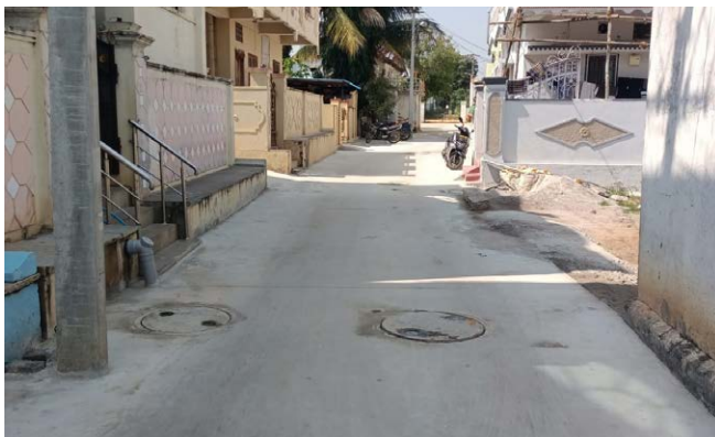
Underground Drainage and other rural development projects in Tangatoor, Shankarpalli near Hyderabad.
